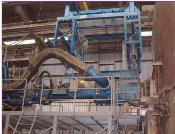
New ROTAFLAM® VERSION 2 in Werk Lengfurt (HeidelbergCement AG)
